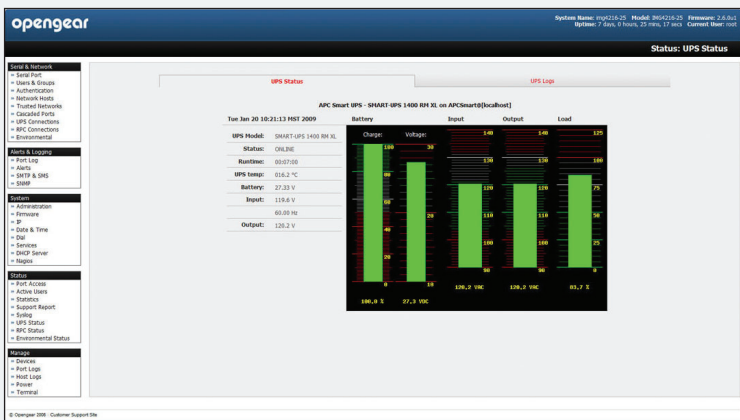
UPS Management: The Opengear NUT Web interface manages system status and logs. UPS status updates monitor battery charge, voltage, input, output, and load.
